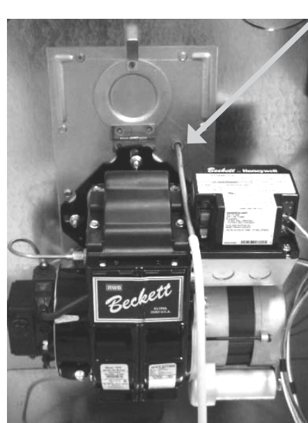
Over-fire draft access port.
